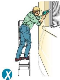
Figure 2a Incorrect - steps side-on to work activity
